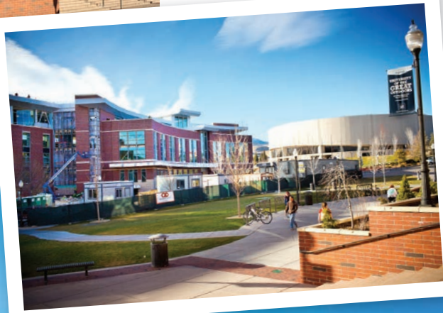
The newly constructed E.L. Wiegand Fitness Center, next to the Lawlor Events Center, is slated to open this spring.
